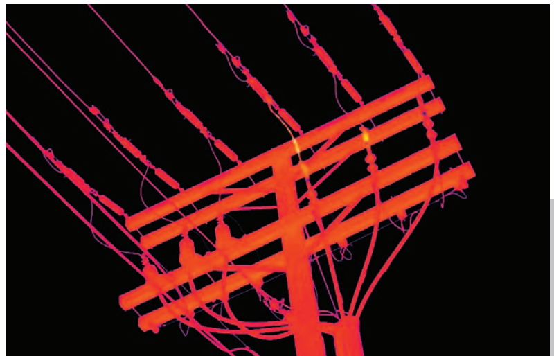
Electrical utility distribution lines
